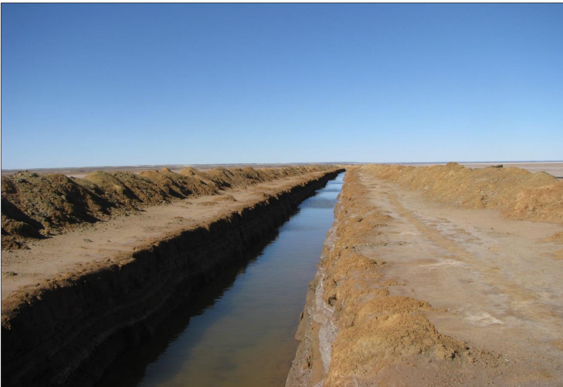
Figure 7,.Close up of trench on Commissioners Pan (Photo Craig Donald Site Plan Consulting)
