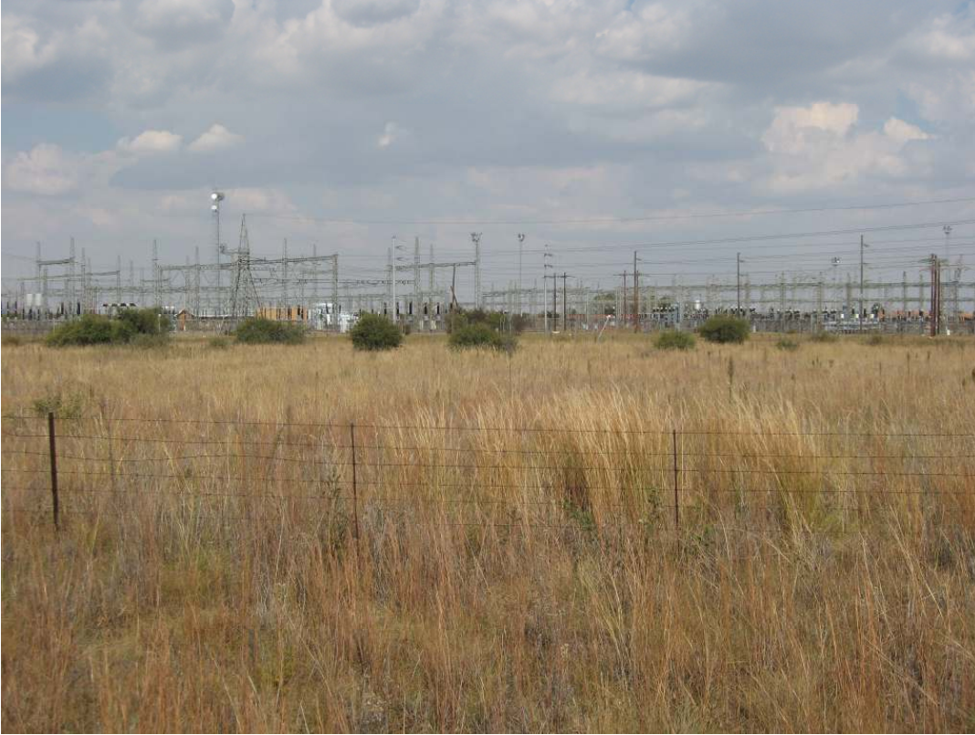
Photo 5: View of the Eskom Watershed substation.
