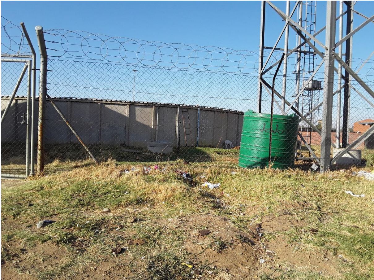
Figure 5 – Water treatment plant in Arlington. GPS coordinates: 28° 01' 35" S 27° 50' 33" E.
