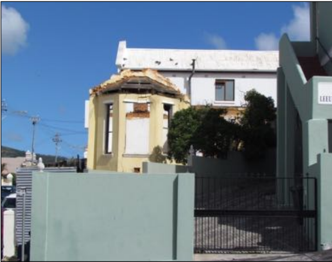
Figure 27: By 2013, the house was a total ruin, with most of the gable and all of the roof gone, and only certain walls remaining standing. (Jim Hislop, 8 March 2013)
