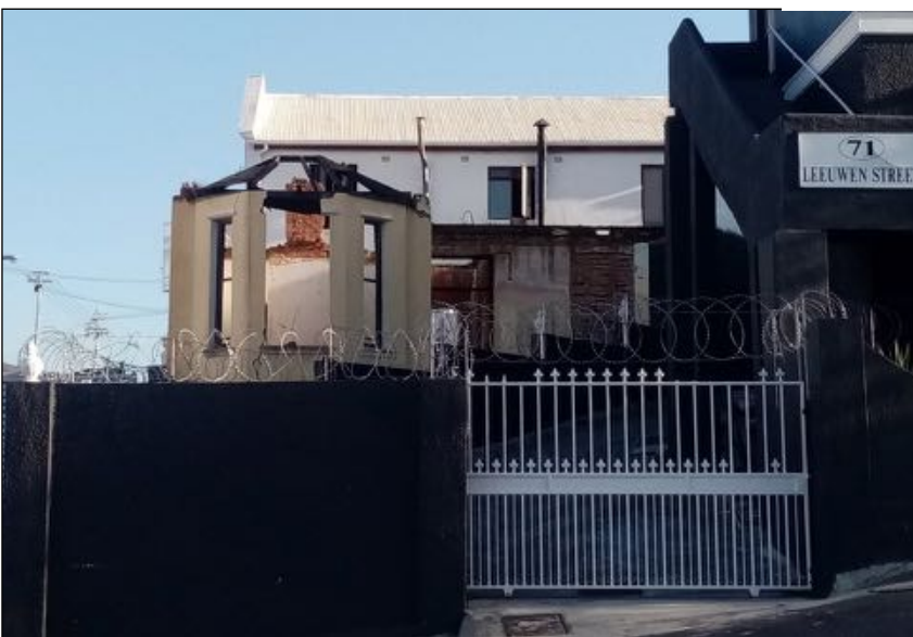
Figure 28: Presently (mid-2020), the bay window roof is missing and the bay window walls are beginning to collapse. (Jim Hislop, 1 June 2020)
