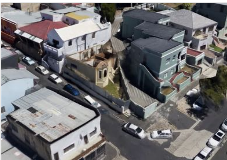
Figure 31: A recent aerial view of the corner of Leeuwen and Lion streets, showing the derelict 2 Lion Street at the centre. Here the steep steep stairs can be seen, as well as the bay windows and internal walls, most of which are still standing. (Google Earth, 2020)
