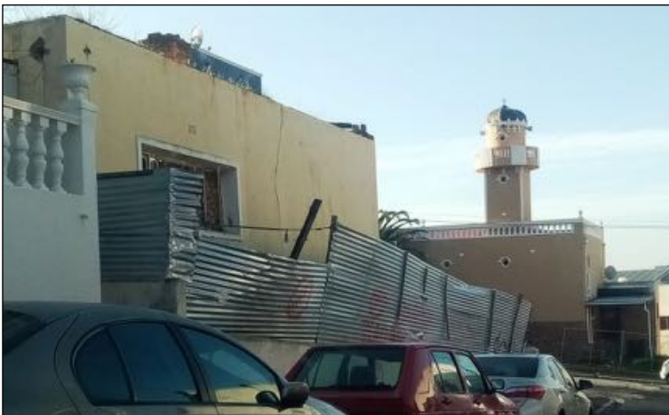
Figure 30: The eastern façade in 2020, showing the remaining eastern wall and steel window that have been bricked up and corrugated iron ‘fencing’ installed in an effort to prevent further vandalism/ degradation of the property. (Jim Hislop, 1 June 2020)
