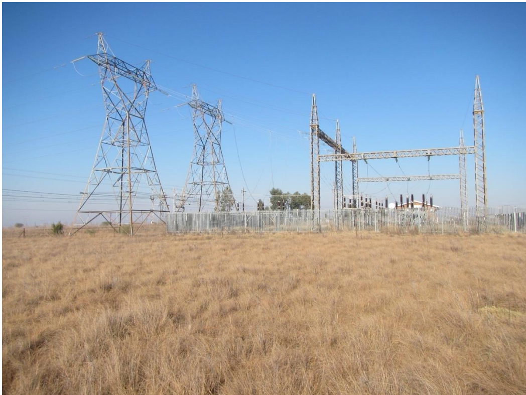
Figure 7: View of existing Substation.
