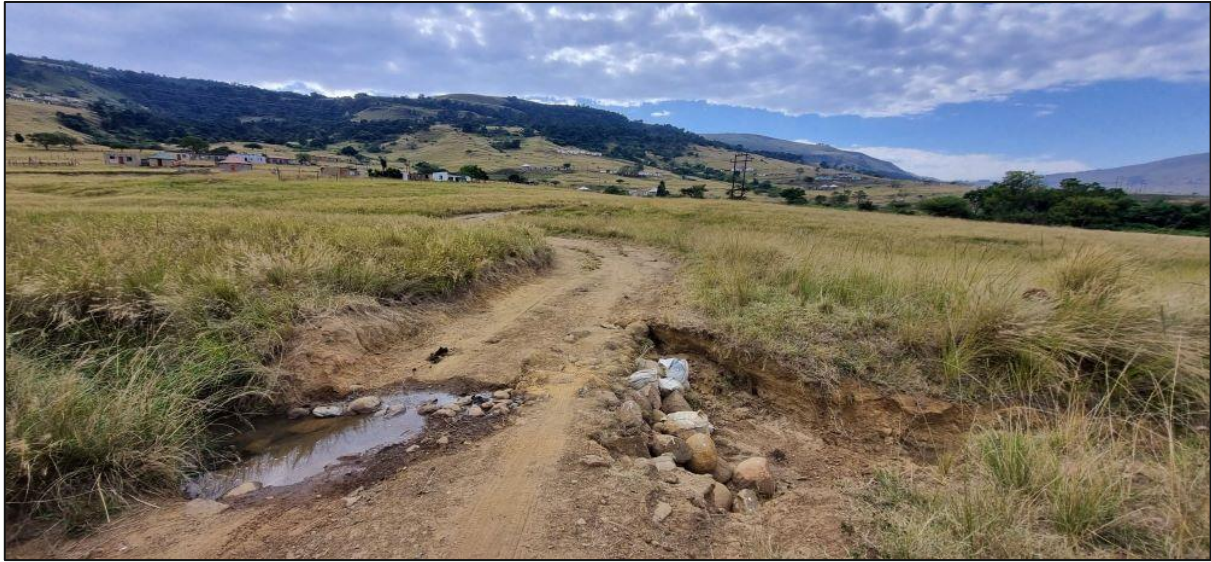
Plate 4: Photograph showing an existing watercourse crossing within the central portion of the route.
