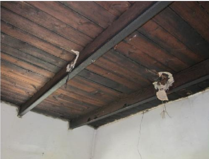
Interior ceiling detail of the original pitched roof structure of the labourer's cottage
