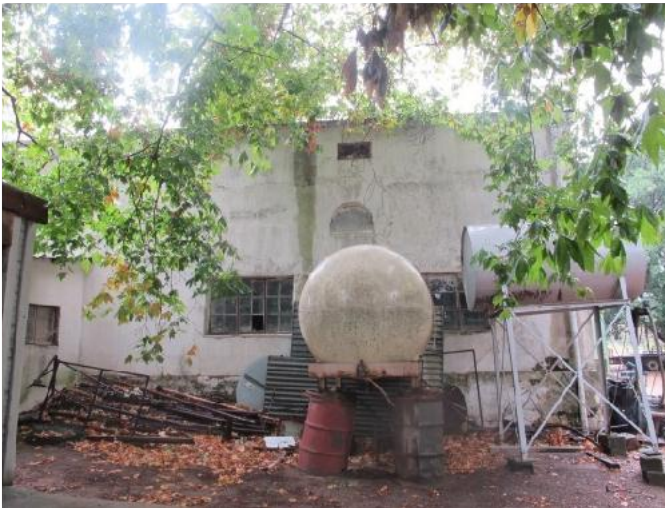
Wine cellar attached to the west end of the farmhouse (north elevation)
