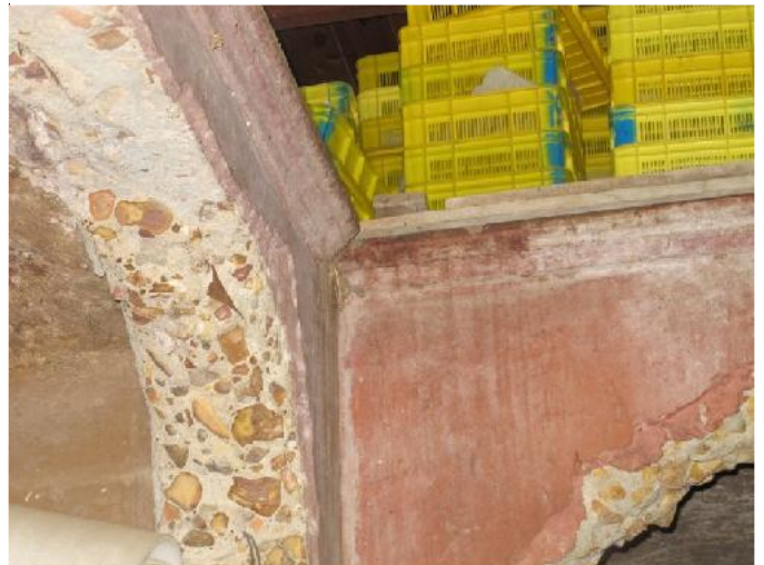
Moulding detail at top of wine tanks. Walls of some tanks have been demolished completely.
