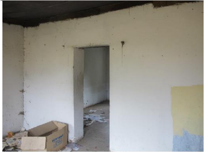
Interior detail of the original pitched roof structure of the labourer's cottage
