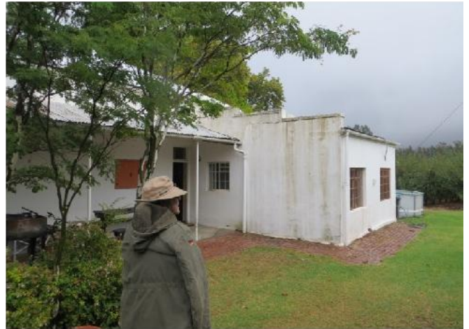
Additional entrance to the east elevation. Accretions clearly detract from the T-shaped building.
