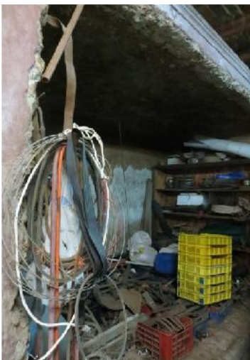
Other tanks have been opened up by demolishing a side wall only
