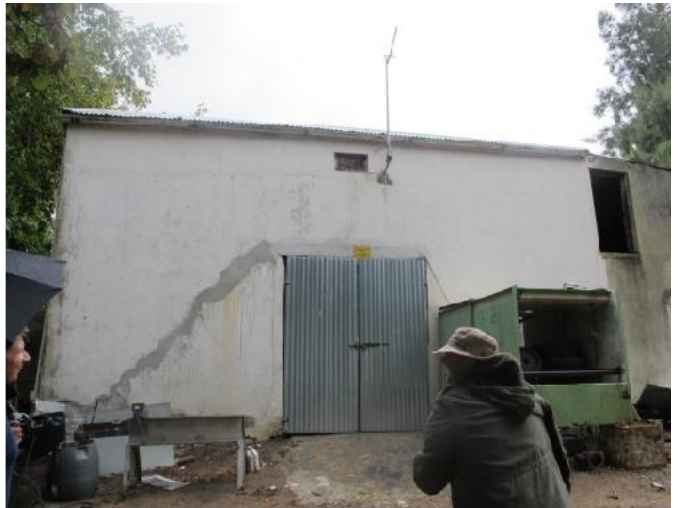
West elevation of cellar attached to farmhouse (c. 1870-80s) facing the outbuilding
