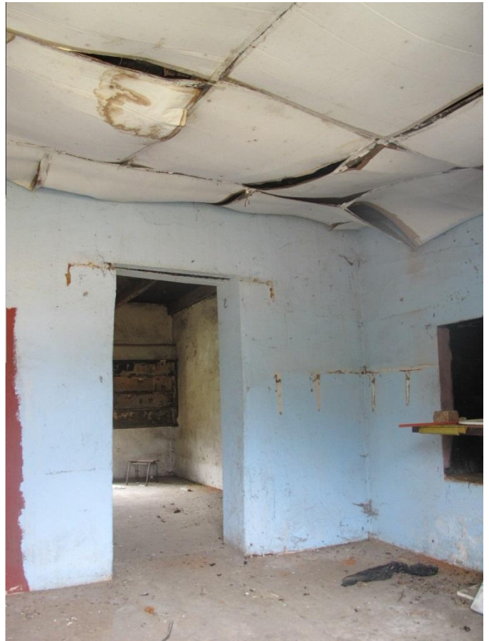
Interior detail of the enclosed stoep addition, with later internal 'hearth' to the right
