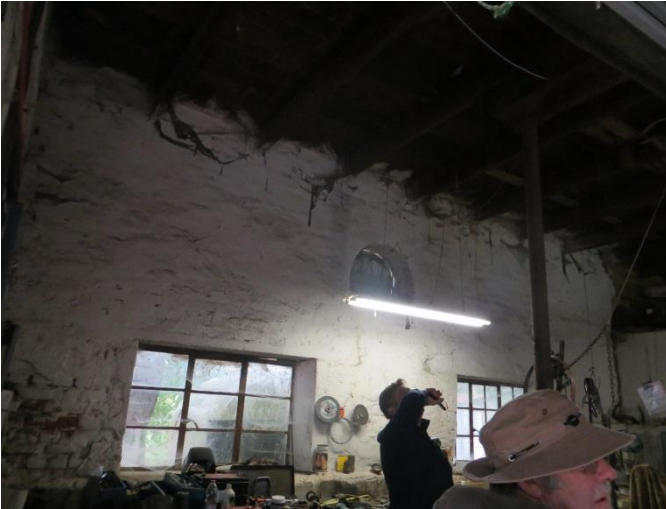
Internal cellar (current workshop). Arched cellar vent opening visible in wall above windows and light
