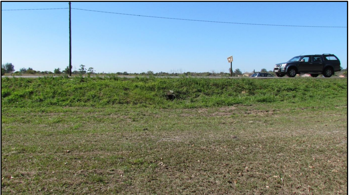
Outlet (W) - Partially Buried
