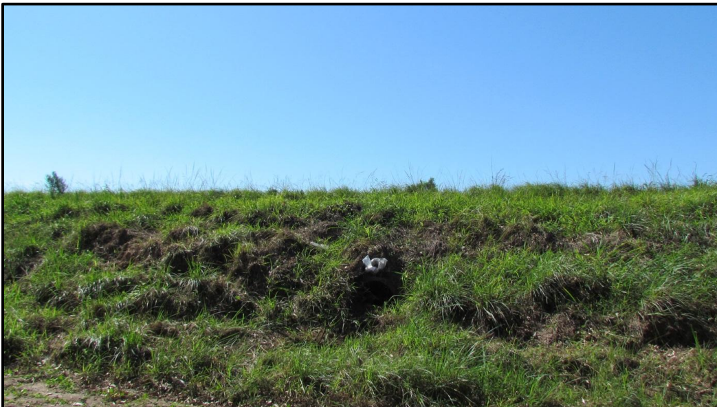
Outlet (W) - Partially buried
