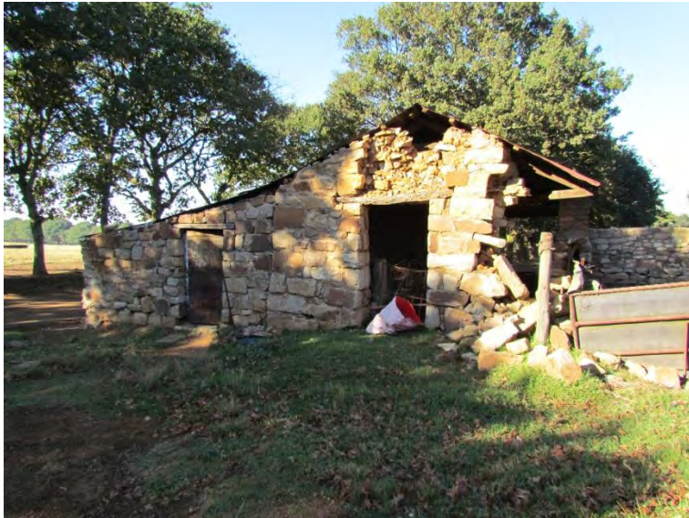
Figure 9-19: The southern elevation of the sandstone stable identified at Site S.36-050. The stable is in a dilapidated state.
