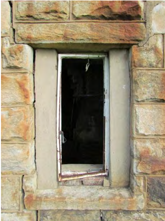
Figure 9-8: The metal window frame on the southern elevation of the house identified at Site S.34-046.
