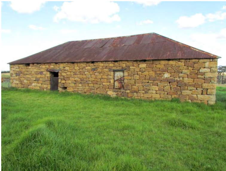
Figure 9-10: The southern elevation of the barn has two windows with wooden frames and corrugated iron doors.
