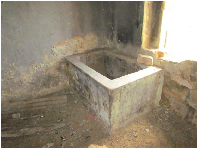
Figure 9-7: Either a bath or a basin identified in the house at Site S.34-046.
