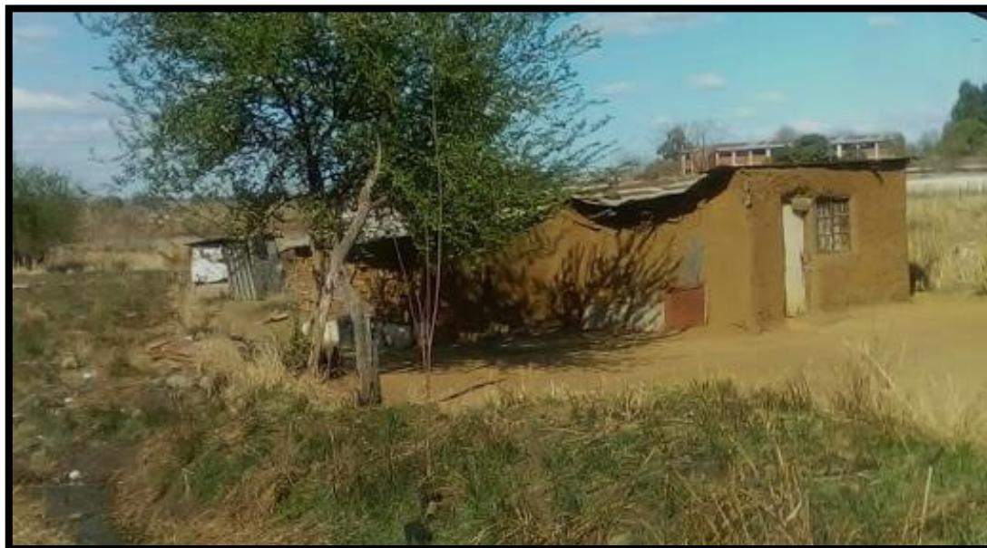
Figure 9. The wattle and daub structure in the north western section of the proposed development plot. This structure is younger than 60 years old and only used as a residence.
