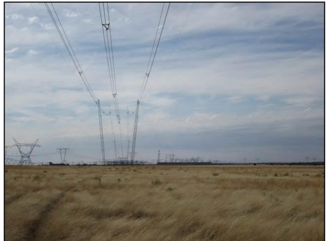
Figure 21: View northwards showing power lines on Braklaagte feeding into Beta Substation.
