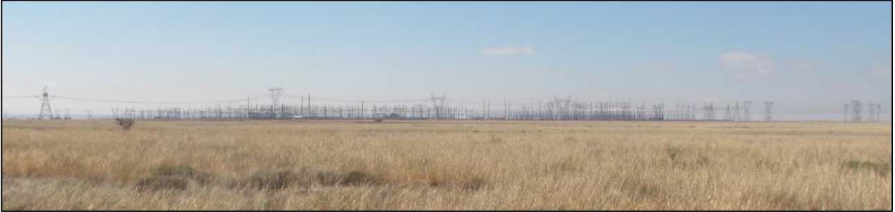
Figure 4: View towards the east from the development area showing the existing Eskom Perseus Substation and associated powerlines.
