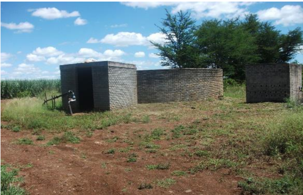
Figure 14: Pump station and reservoir
