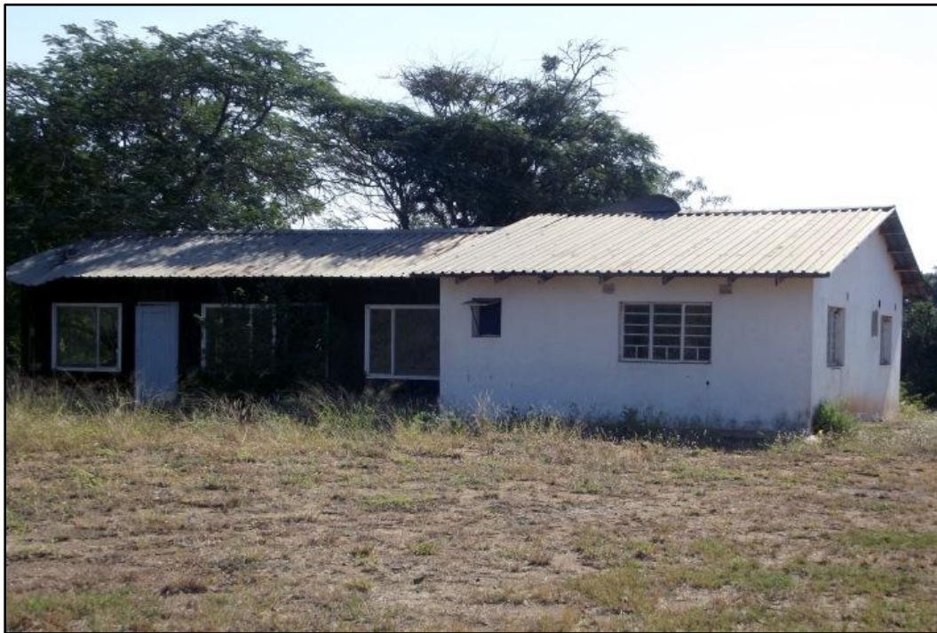
Fig. 31. Site MF 17. Old farm offices. Approaching 60 years of age. Photo taken west.
