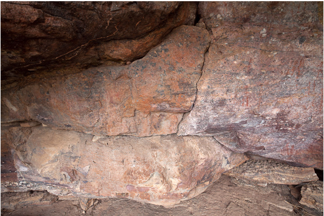
Figure 11. Left hand side of Mdoni Shelter. Located at the upstream end of the shelter, this area has suffered chemical weathering in the form of what may be mineral salt-laden water within the rock that has left a white deposit on the rock that obscures the few paintings here. Mdoni Panel A is on the left and part of Panel B is on the right
