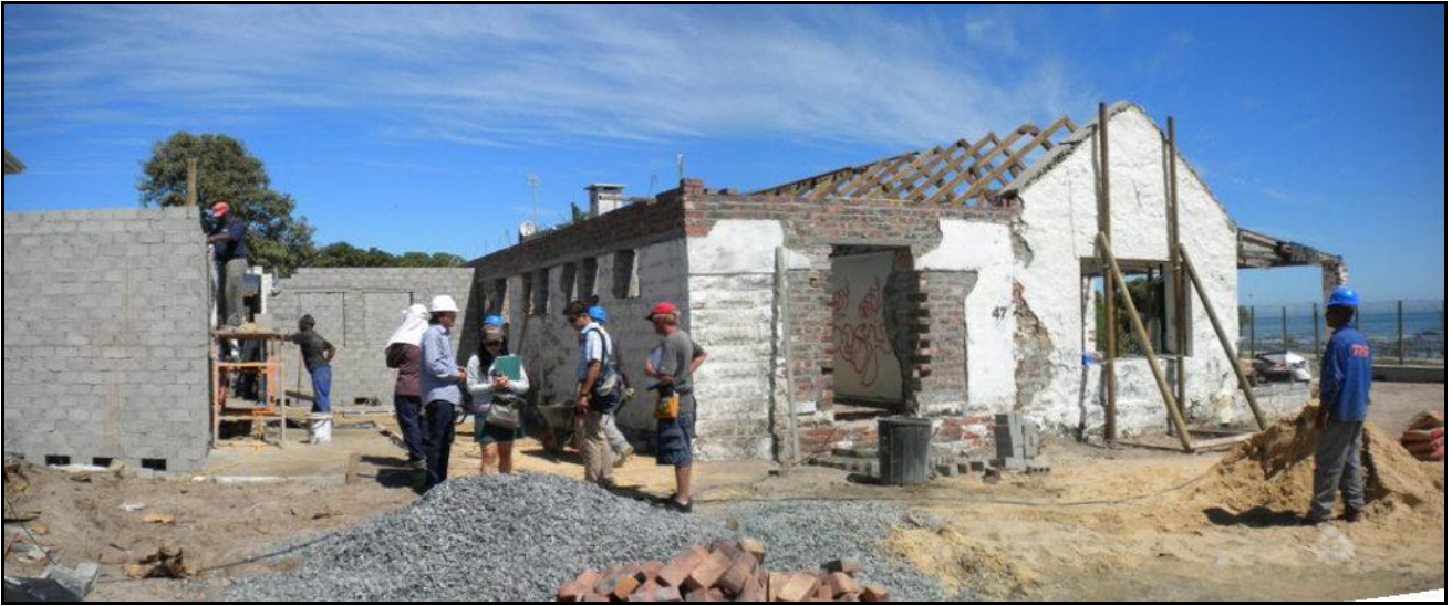
Figure 3: View towards the south showing the disturbed yard. This photograph (provided by Heritage Western Cape) was taken on 11 th March 2010 before we were called to site.
