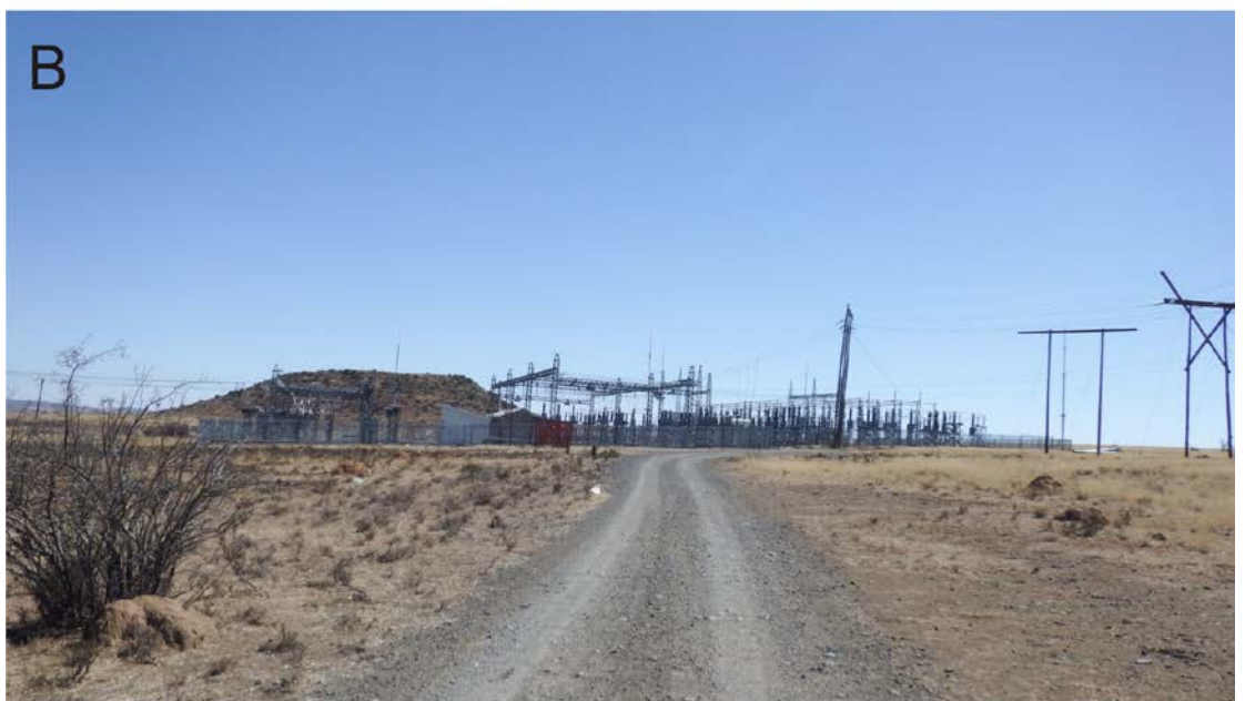
Figure 10. General view of the footprint near its connection point with the Melkspruit Substation (below).
