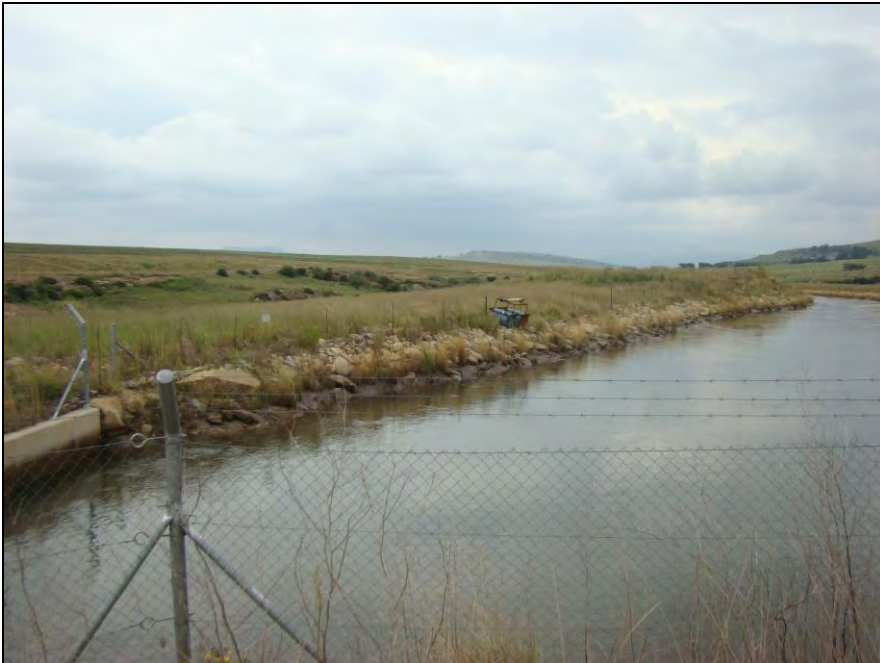
Fig.11 Point C on the water extraction channel at Marino 1487, Bethlehem along the Asrivier.
