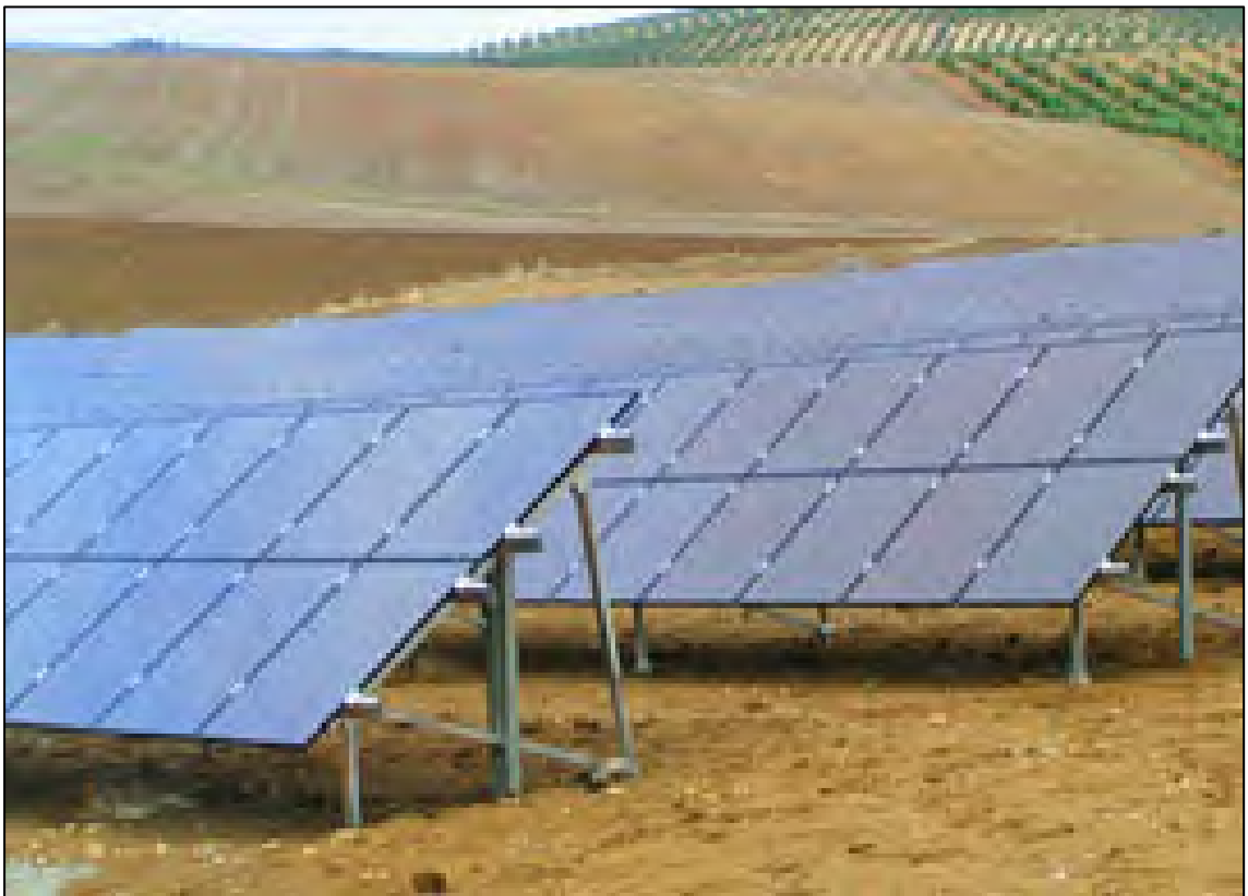
Figure 2: An Example of a Photovoltaic Power Plant
