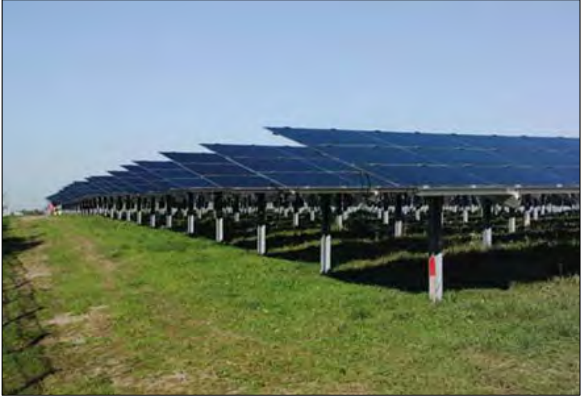
Figure 1: An Example of a Photovoltaic Power Plant
