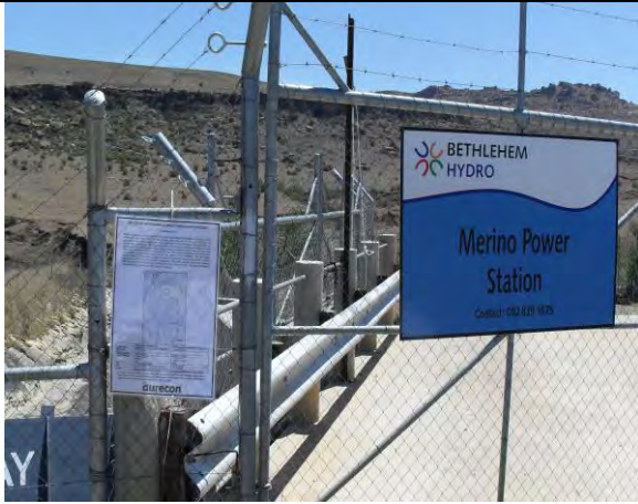
Photo 11: Notice of EA attached to the fence at the intake canal at the Bethlehem Hydro
