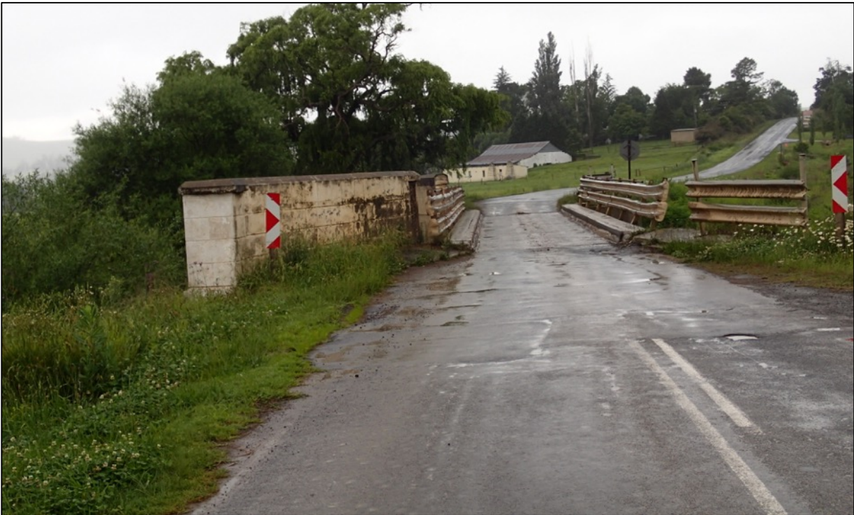
Figure 4. The Current state of the Meshlyn Bridge
