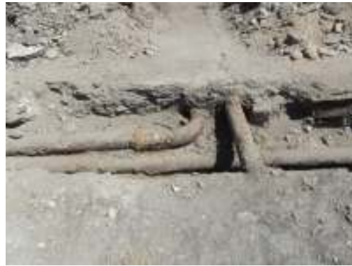
Figure 13: Rusty pipes in trench.
