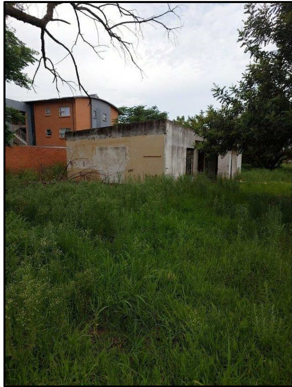
Figure 7.6. Small labourer's house situated along the western edge of the proposed project area South facing wall.
