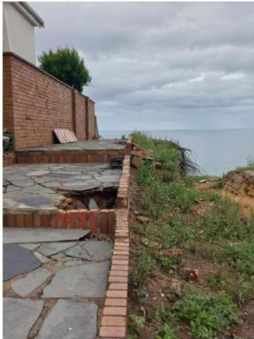
SLIDE 4 : VISUALS OF HISTORICAL DAMAGE TO NEIGHBOUR'S BOUNDARY WALL
