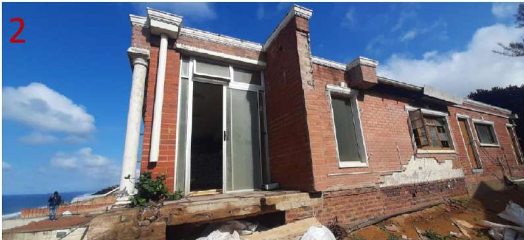
North-East Elevation of existing house with illegal additions, damaged walls with collapsing brick faggot façade
