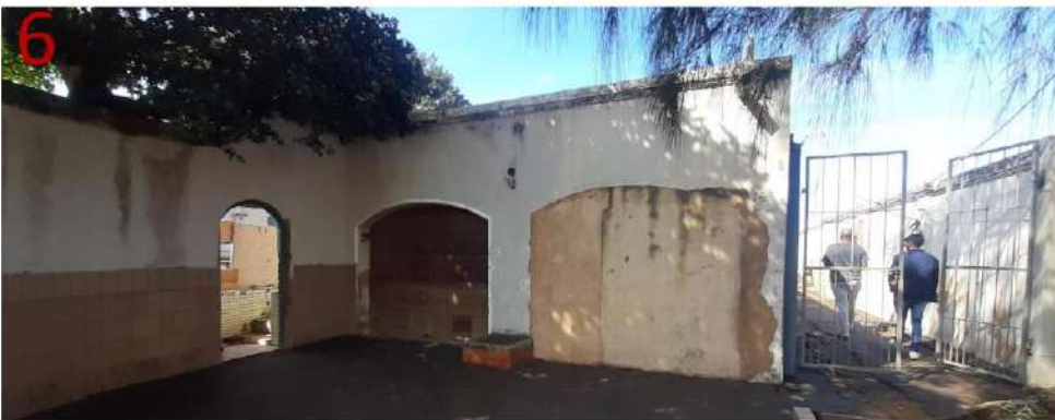
North-West façade of existing outbuilding, screening wall and boundary wall with illegal alterations
