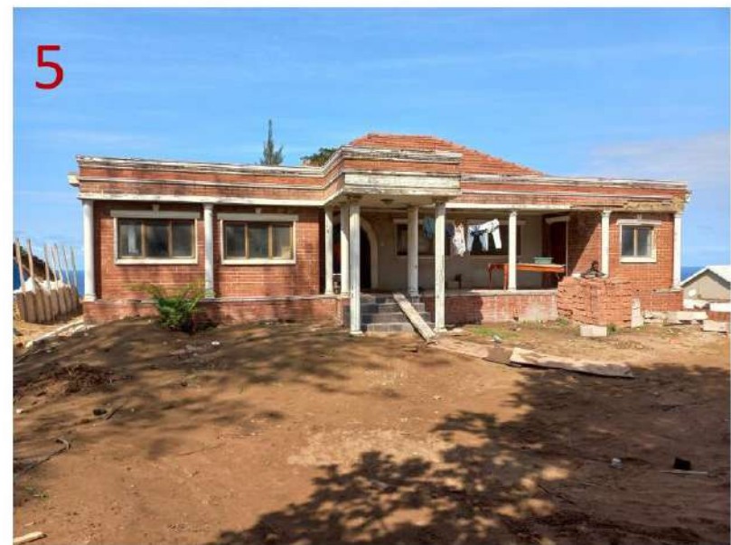
North-West façade of existing house representing illegal alterations, dwelling extensions poor condition of structure and site soil
