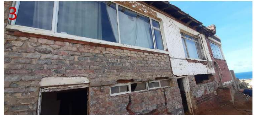
Section of South-West Elevation of existing house with illegal additions, and room extension. Structural integrity compromised as shown by severe cracks on walls
