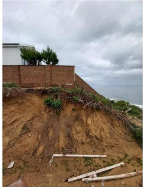
SLIDE 2 : DAMAGE ALONG THE NORTH EASTERN CORNER
