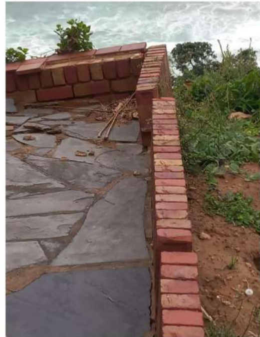
SLIDE 5 : VISUALS OF HISTORICAL DAMAGE TO NEIGHBOUR'S BOUNDARY WALL
