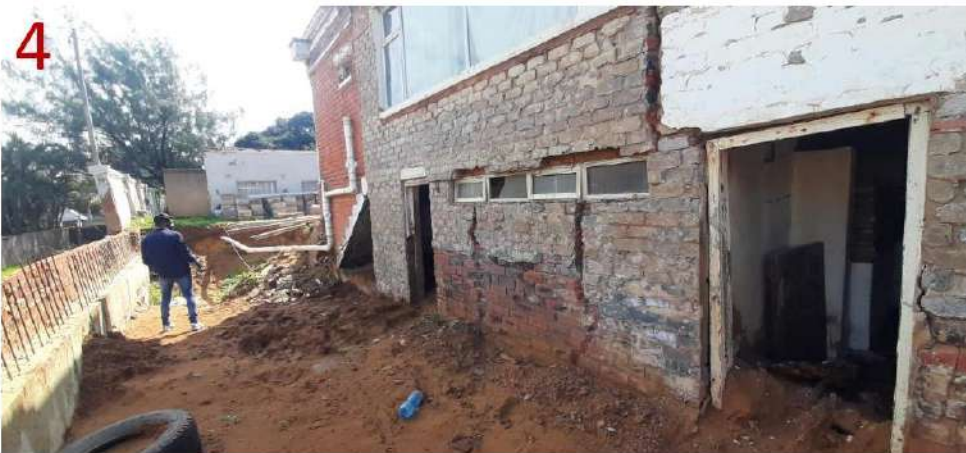
Section of South-West Elevation of existing house with illegal additions, and room extension. Structural integrity compromised as shown by severe cracks on walls
