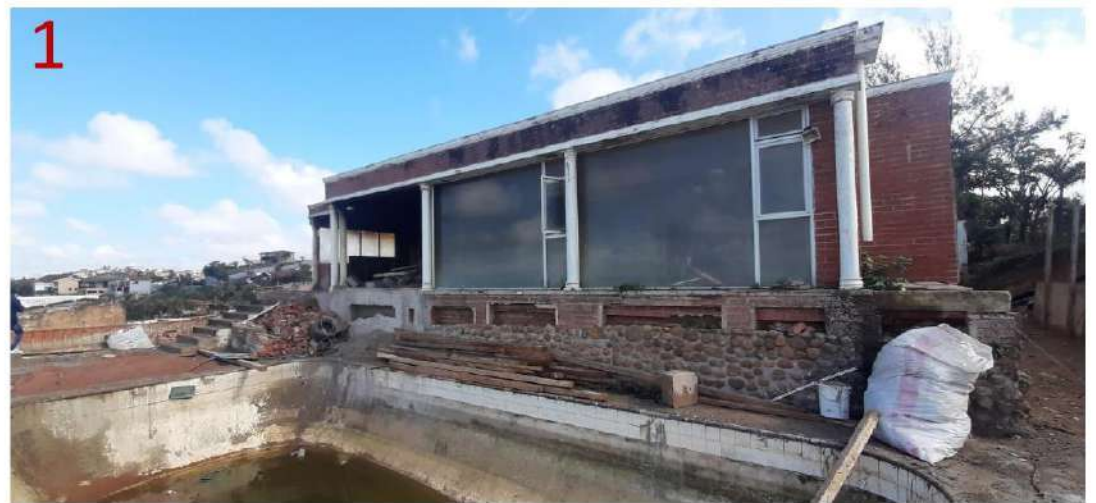
South-East façade of existing house representing illegal alterations and deteriorating condition of structure
