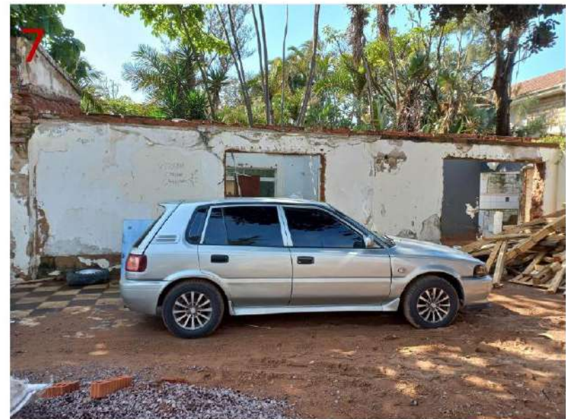
South-West elevation of existing nursery rooms and water closets representing poor condition of structure
