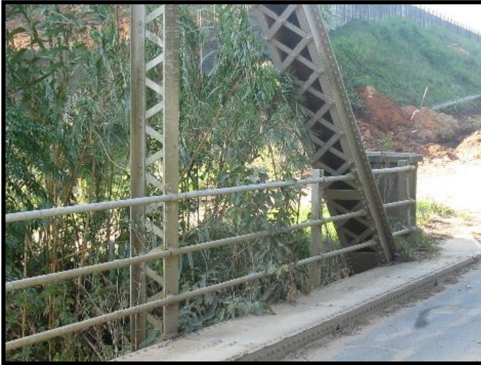
Figure 12. The steel bridge across the Mtwalume River may be older than 60 years old. However it is situated more than 100m from the project area at S 30 28' 39.07" E 30 36' 23.82" and is not threatened by the proposed development.
