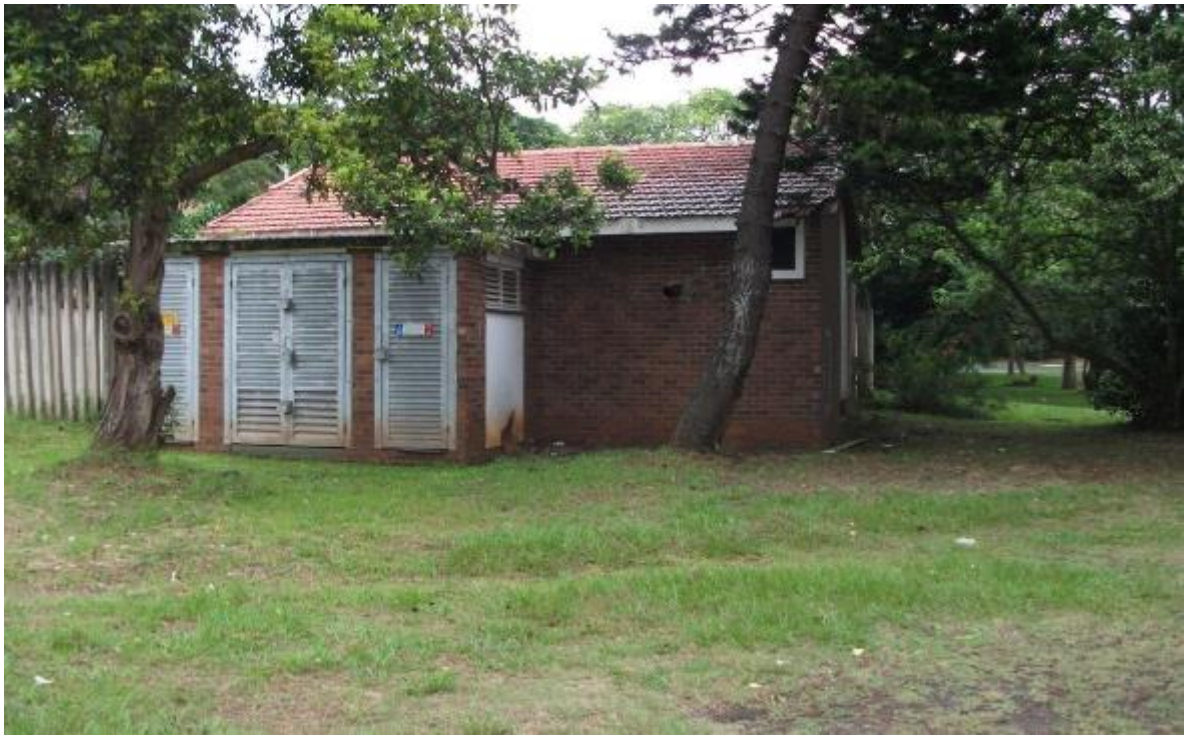
Figure 14: Municipal water treatment plant
