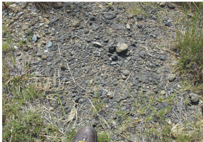
Figure 12. Area 1; road gravel and chunks of tar litter the veld on the southern side of the bridge.
