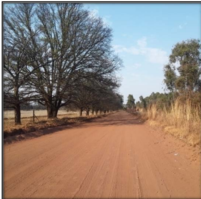
Figure 21: Starting point of the NBC Road re-alignment (D2809) GPS coordinates 25.712778S 30.042778E
