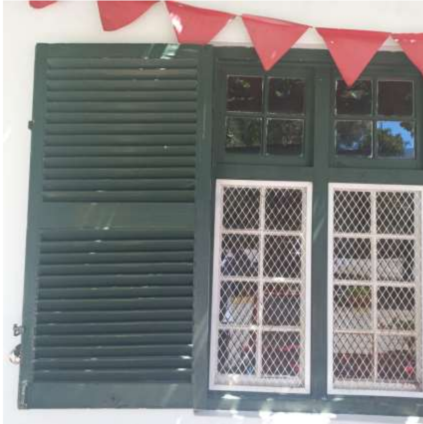
Photo 48. A closer view of the windows the building, and their shutters. These are most likely the original windows. Photo: Adolfo Linares.
