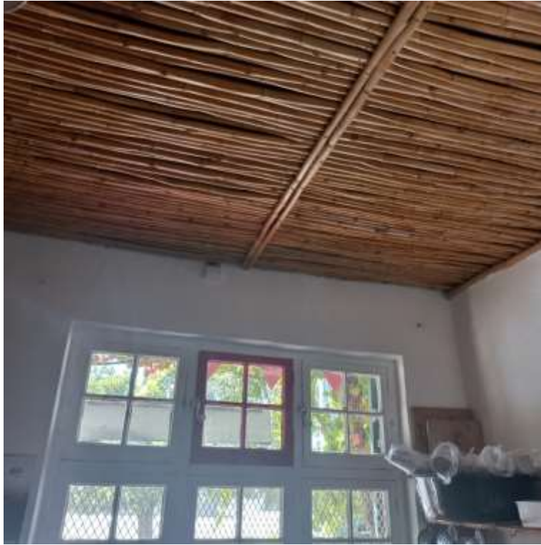
Photo 49. An interior view of the original windows, and of the reed ceiling. Photo: Adolfo Linares.
