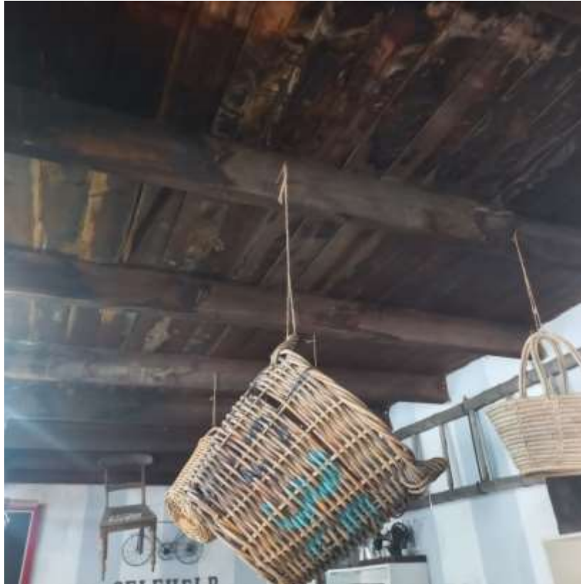
Photo 51. The original wooden ceiling of the building is clearly very old, and is much stained and weathered. Photo: Adolfo Linares.
