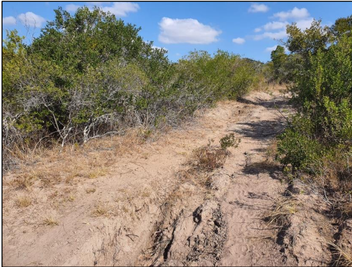
Figure 4-7: View of the highly eroded existing access road to Ncera in the project area.
