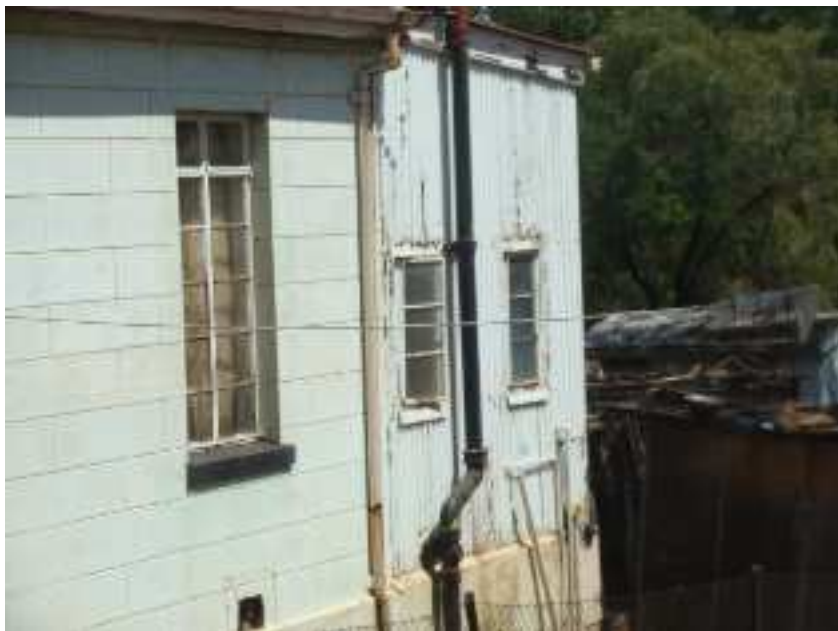
Figure 13: A number of houses in the area contain these corrugated iron additions that could also be older than 60 years of age.
