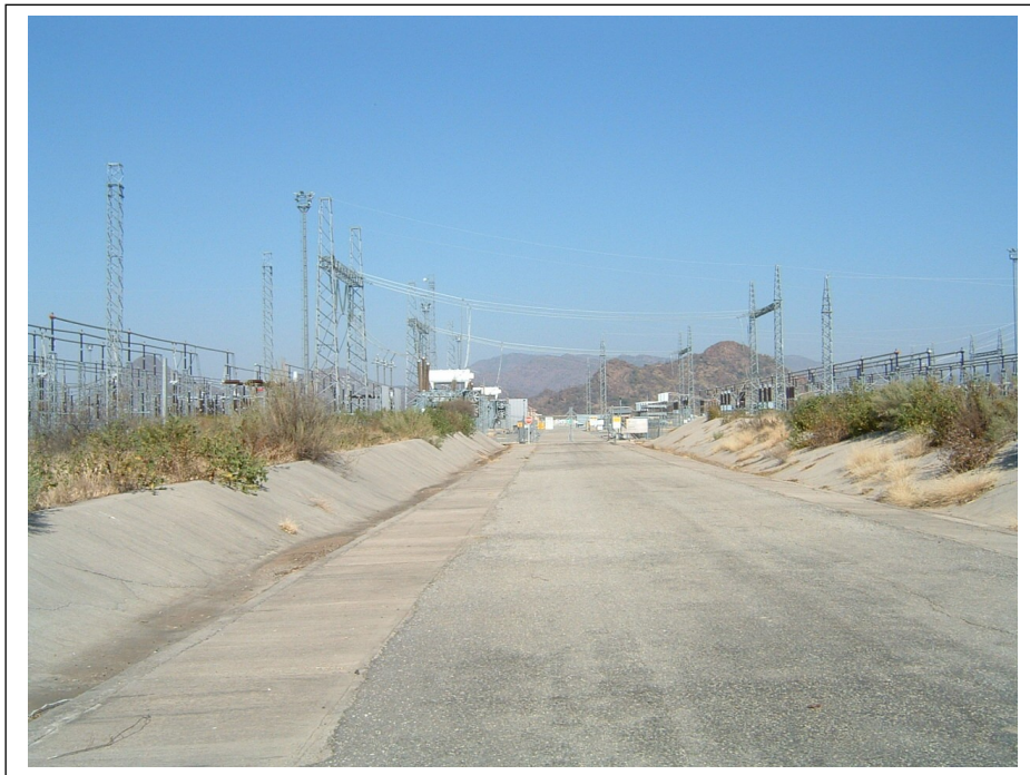
Figure 7 – Alternative 01 and Alternative 02 broadly follows the same power line corridor, except for a short stretch towards the end of the power line before entering the Leseding Substation on the farm Hackney 115KT (above).
