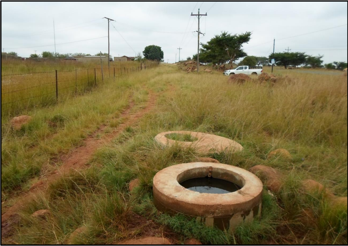
Figure 5: Manholes marking the existing pipeline.
