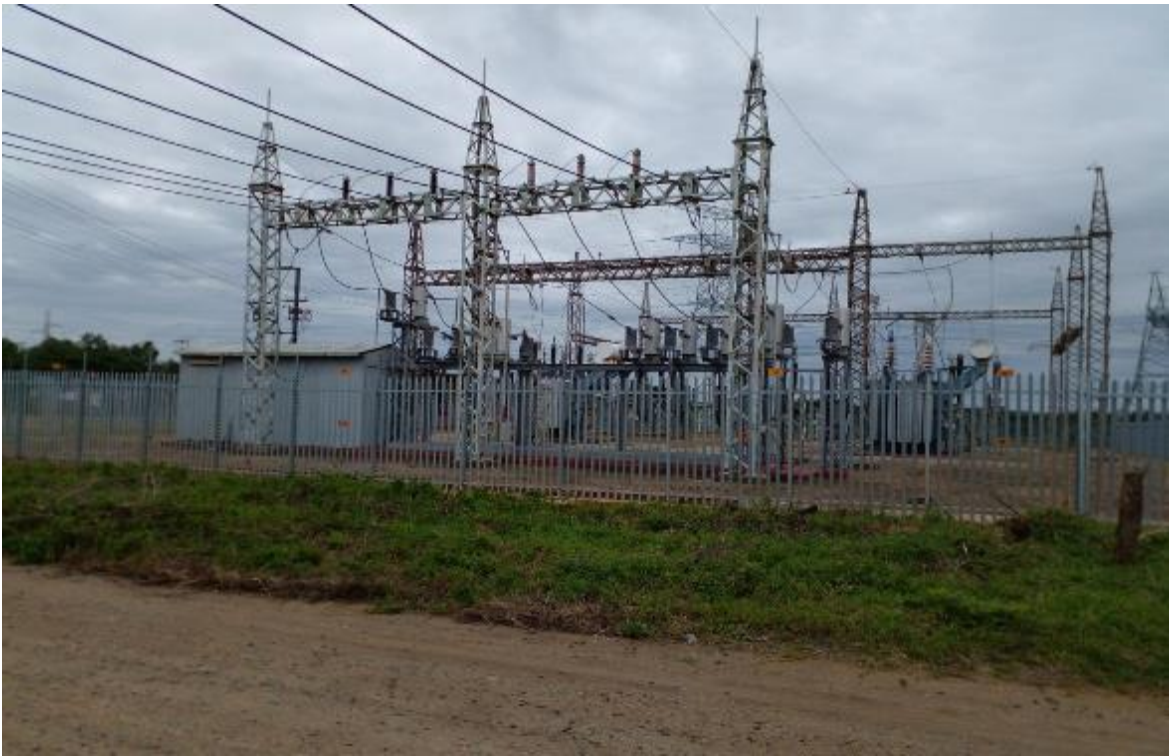
Figure 14: Substation with pipeline route between substation and road
