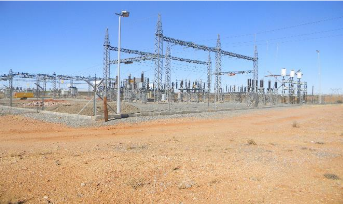
Plate 1: Photo 1: View of Oasis Substation where the powerline development starts (Photograph © by Author 2017).
