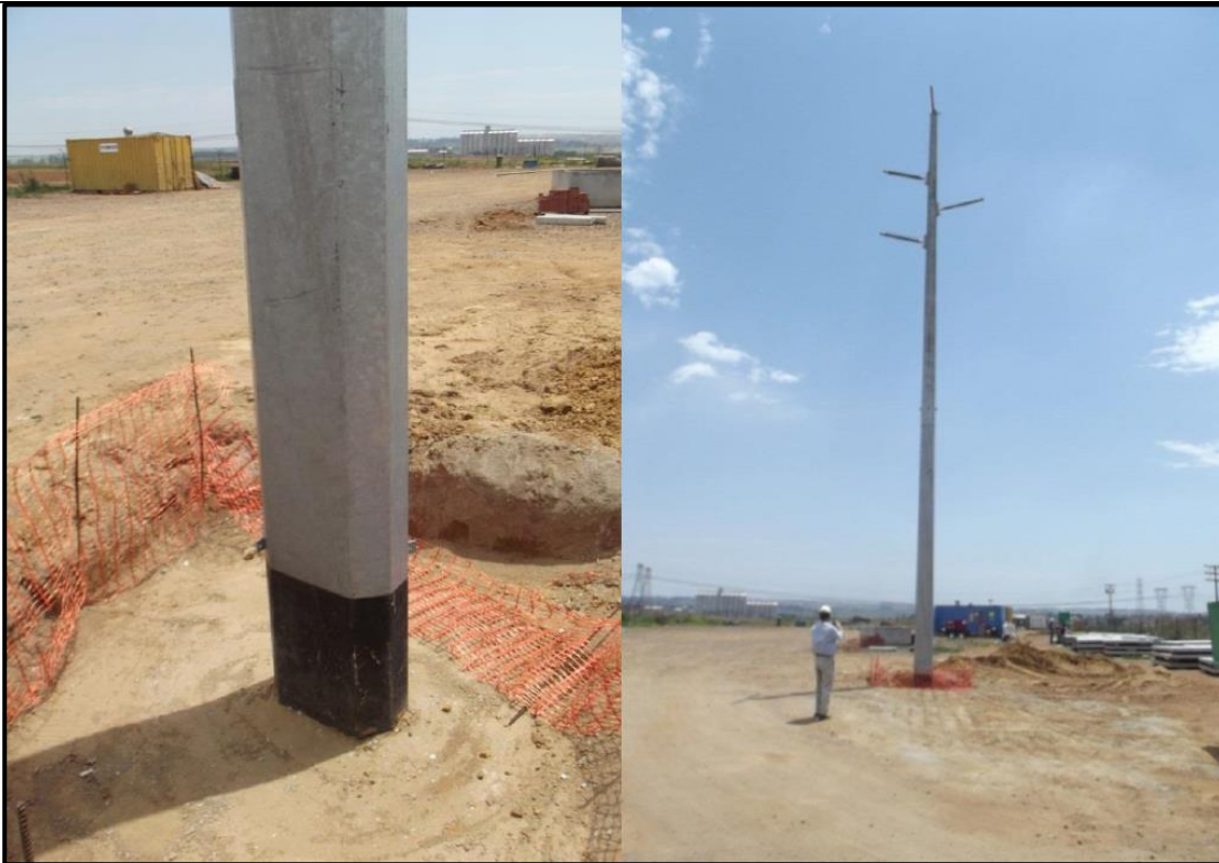
Figure 4: Example of Steel Mono-Pole Type to replace the existing 5-pole wooden pylons
