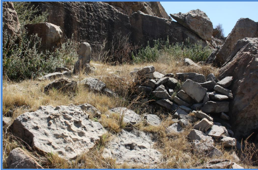
Plate 03: View of the section of the collapsed stone wall
