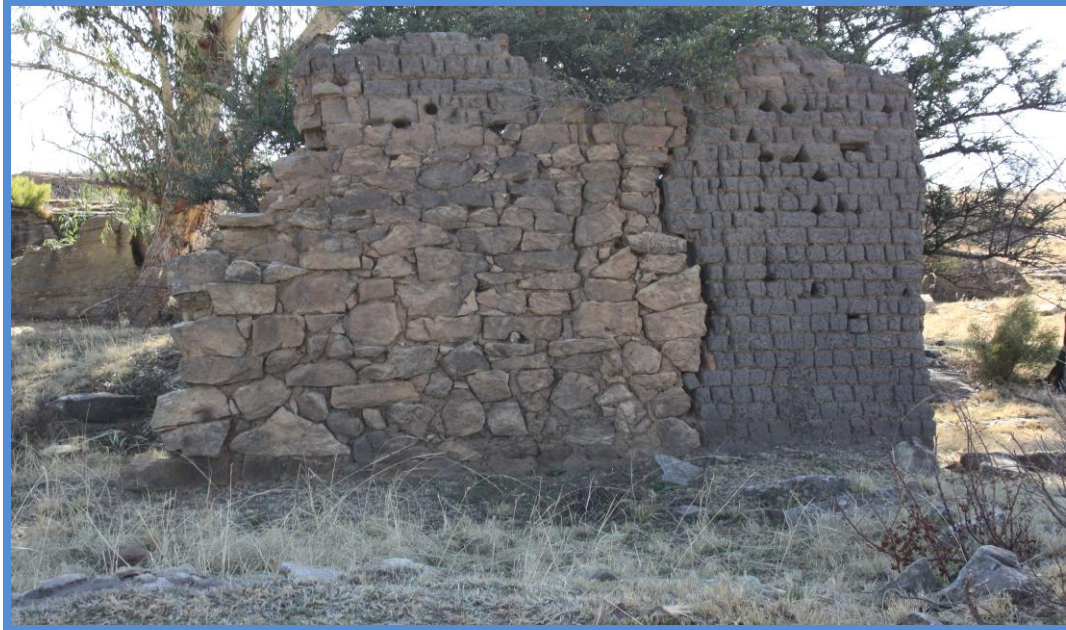
Plate 20: View of the dilapidated house represented by a free standing wall showing two types of construction techniques.
