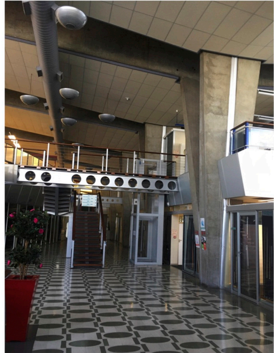
Ocean Terminal, Double volumes internal passage Image shows broad, split columns supporting the folded concrete roof slab Terazzo floor tiles from original
