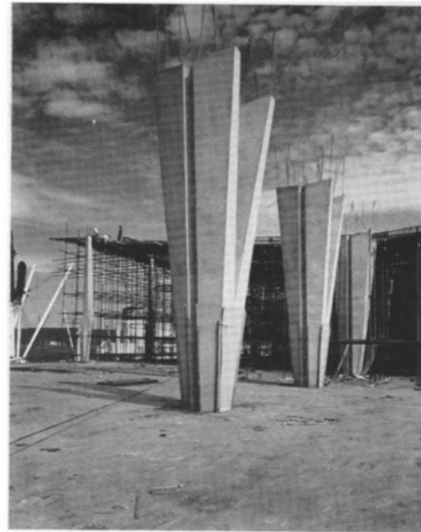
Central columns of the concourse are precast and give a sculpture-like effect
