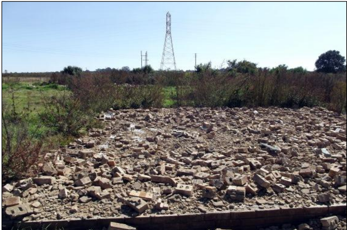
Fig. 16. Site OG 14. One of the seven demolished houses at this site. Photo taken in western direction.
