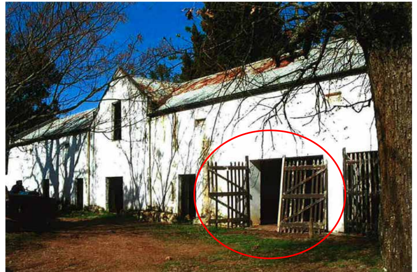
Figure 18. Front elevation with slatted garage doors; detail of shutters (indicated in red) to be replicated and reinstated (Image: Vos 2011)
