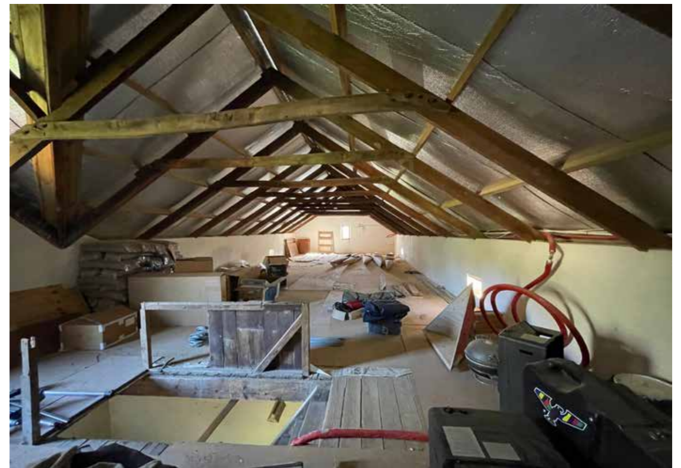
Figure 12. Open attic space with central gable and end gable windows (Image: RSA 2023)
