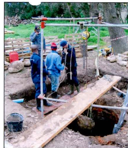
Plate 2: A chain block was used for removing large rocks from the well and seeping water was pumped out.
