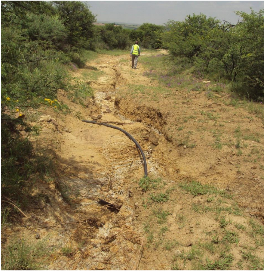
Figure 8: View of a heavily eroded farm road in the north-western section of the project footprint
