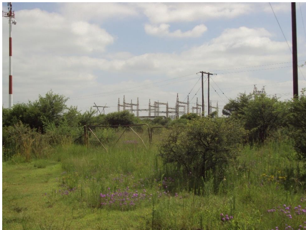
Figure 7: View of the existing electrical substation situated on the northern section of the Oslaagte Solar 1 footprint, note the dense acacia thicket surrounding the substation
