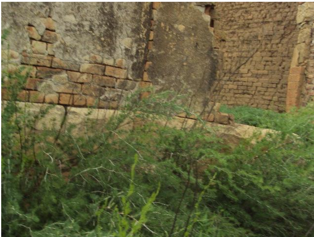
Figure 51: View of the farmhouse construction materials; showing sandstone foundation, mud bricks and commercial bricks
