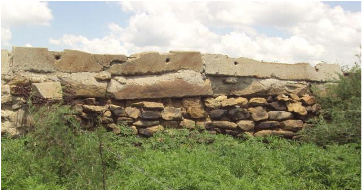
Figure 55: View of kraal wall, showing past repair work
