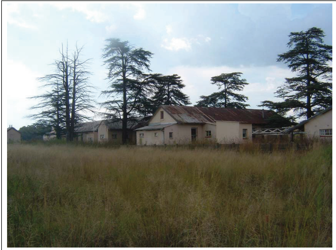
Figure 4- The abandoned mine hospital incorporates a number of buildings which are currently being vandalised as buildings are stripped for building material and features such as doors and window frames (above).
