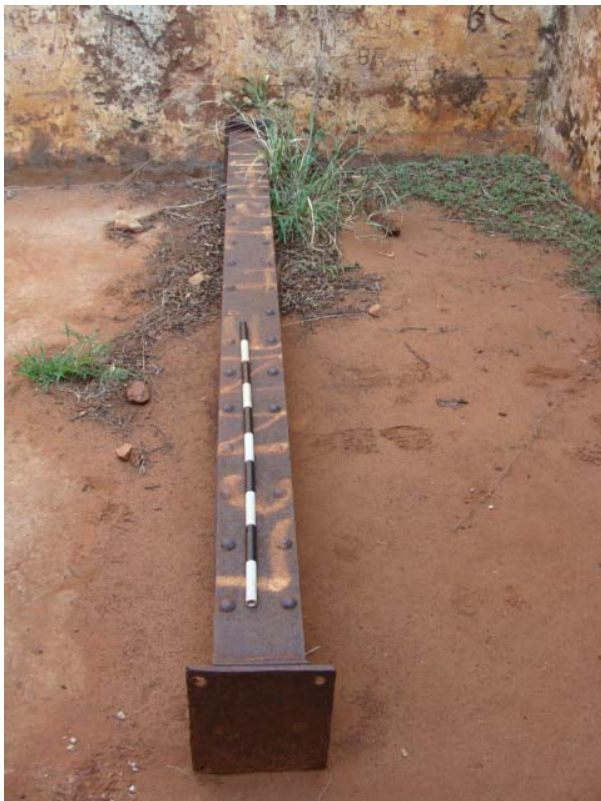
Figure 130 Loose steel pillar in one of the rooms of the fort.
