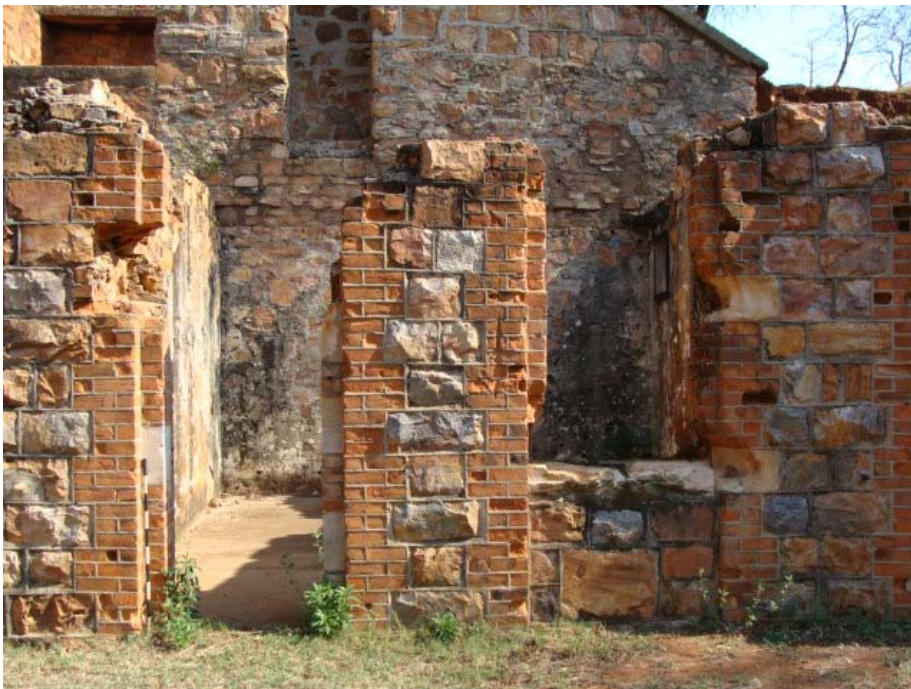
Figure 122 Front view of the telegraph room.
