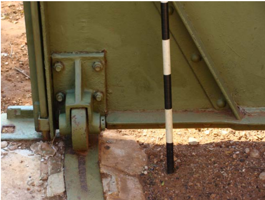
Figure 86 Wheel on which the steel doors of the fort slide into position.
