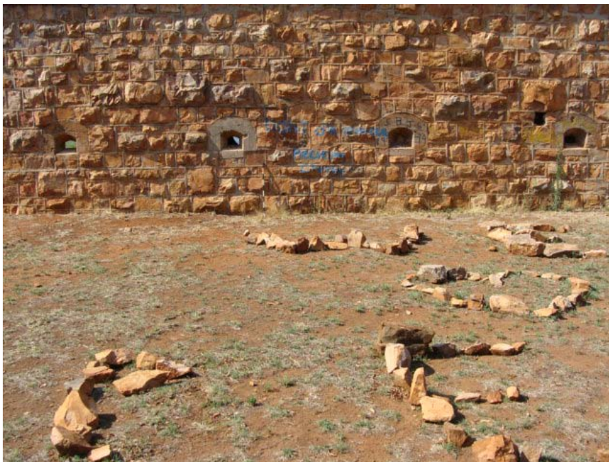
Figure 94 Graffiti against the inside wall of the fort and packed stones in the courtyard indicating recent activities damaging the site.
