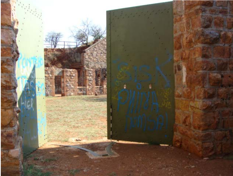
Figure 87 Second set of entrance doors to the fort. Note the very recent graffiti which can also be seen on other parts of the fort.
