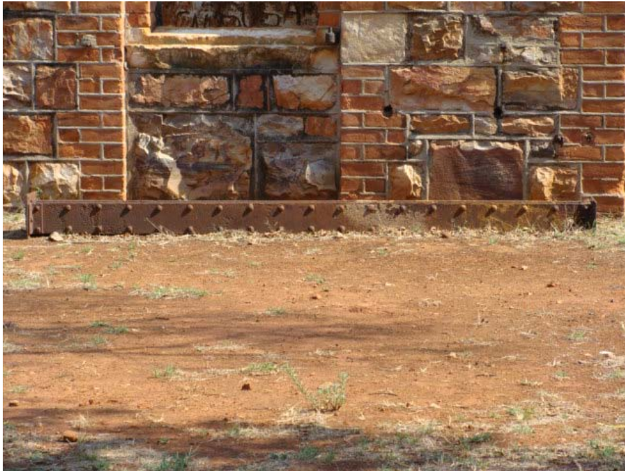
Figure 129 Loose steel pillar in the courtyard.
