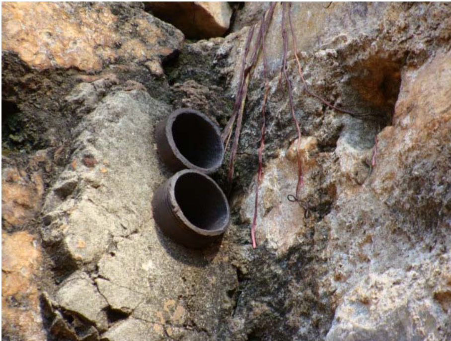
Figure 146 Metal pipes used to protect the electricity wiring of the fort.
