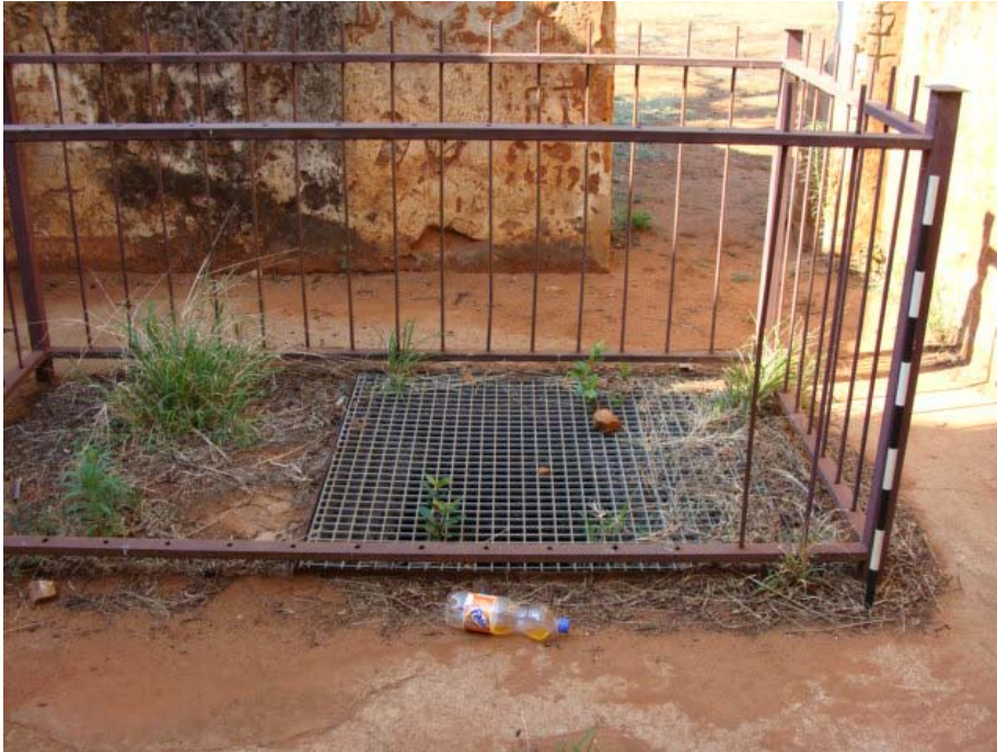
Figure 133 Close-up view of the broken barrier at the water reservoir.
