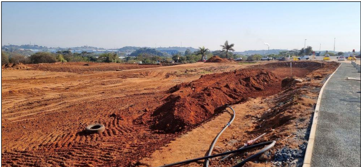
Plate 2: Photograph showing the access road to the site which is in the process of being widened.
