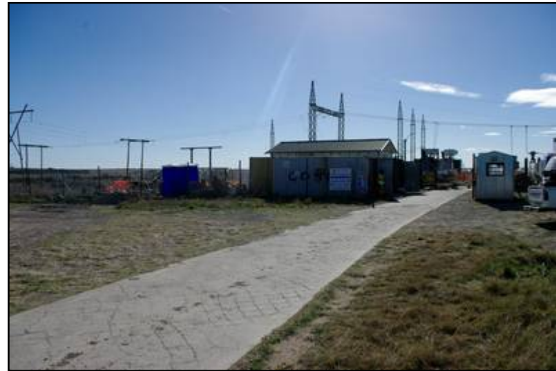
Plate 8: View of the Chaba substation
