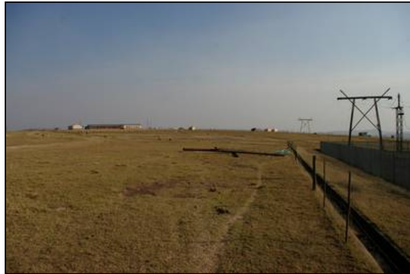
Plate 16: View of the Tyalra to Qunu line route from the Qunu substation
