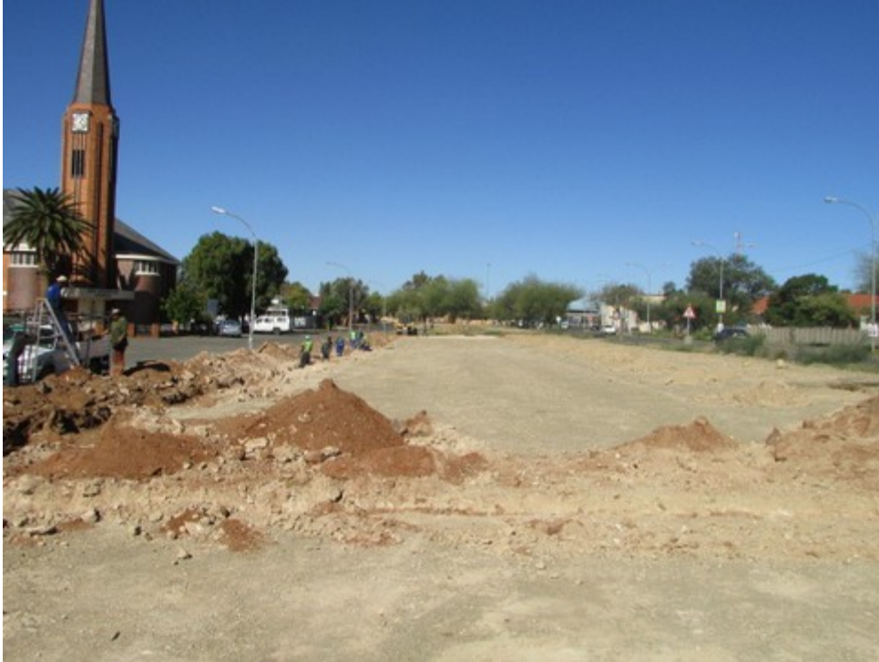
Figure 2: The development area taken from Lawrence street towards the east showing the foundations test trenches being dug.
