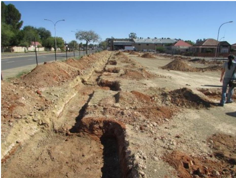
Figure 3: A closer view of the foundation trenches taken down Quinn street towards Lawrence street.
