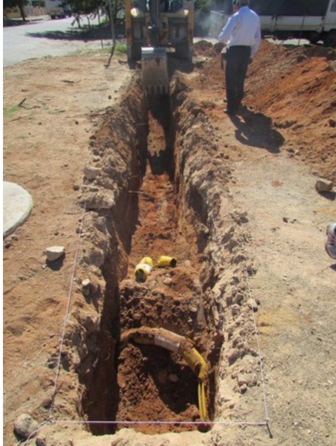
Figure 8: TT1 being excavated. A section of the Neotel Line connection was exposed.
