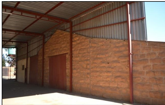
Figure 19. Old sandstone shed - one of the former dwellings now incorporated into the a new steel frame shed structure
