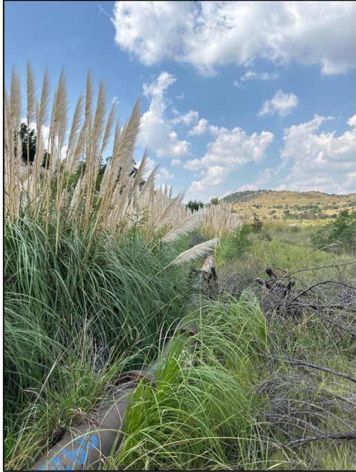
Figure 13 – View of the existing pipeline in the northern part of the study area.
