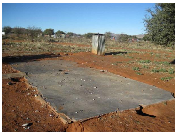
Figure 17 – Foundations and remains of informal housing
