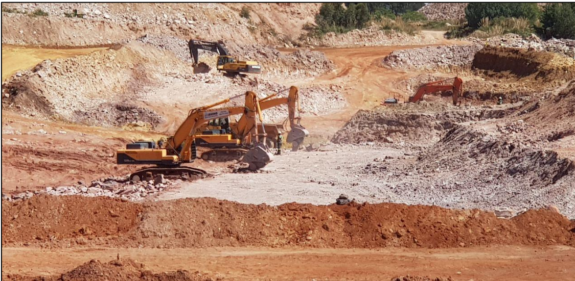
Figure 5: Closer view of the equipment used to break up the rock. The machine uses an Xcentric Ripper, which is an attachment developed for high-performance rock excavation and concrete demolition work. The production rates are up to 5 times greater than using a hydraulic breaker.
