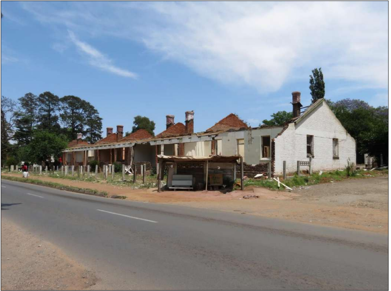
Figure 133 – General view of Building Type 27 as seen during the site visit of Tuesday, 28 October 2014.
