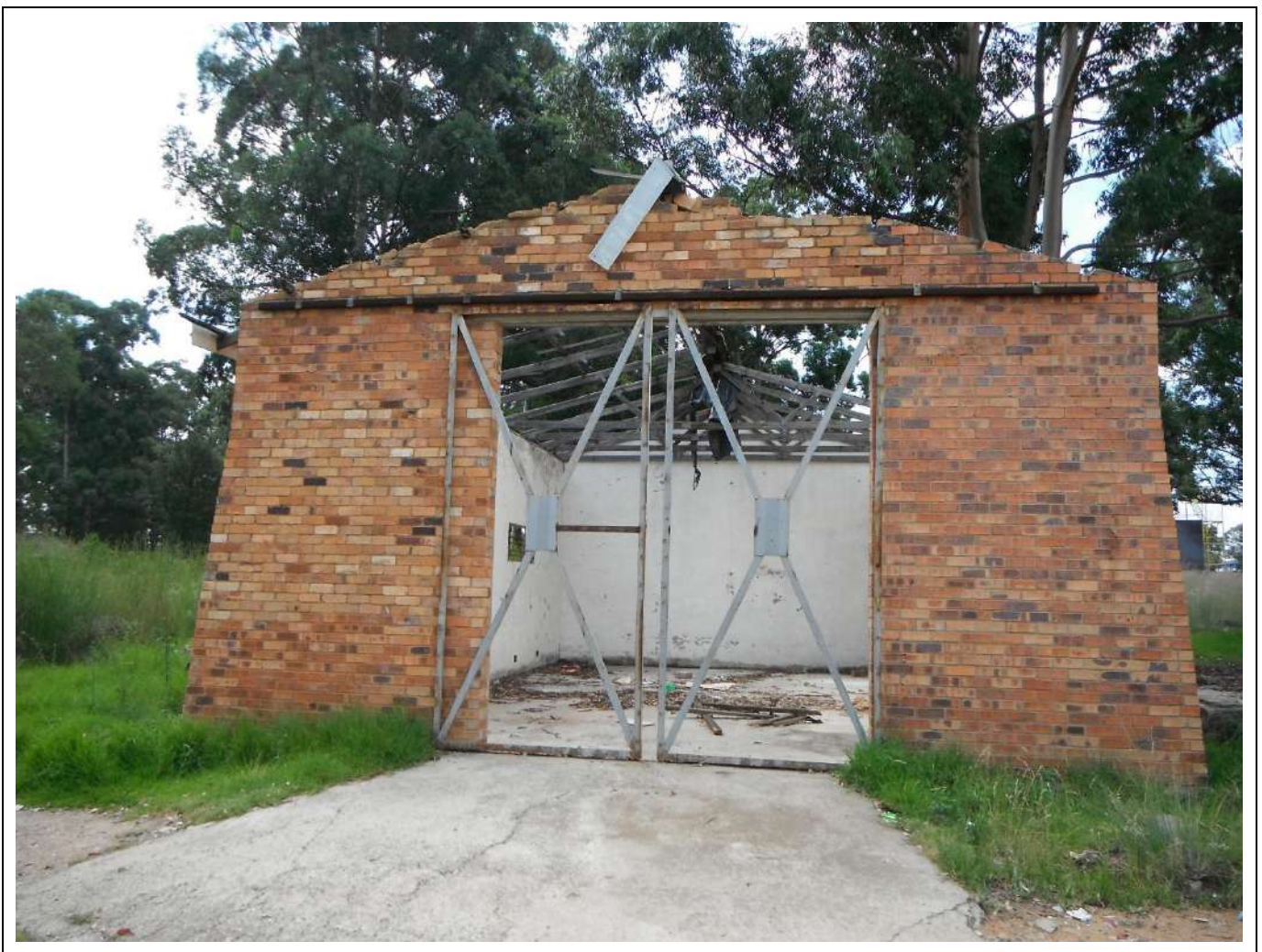
Figure 93 – General view of the Building Type 14 structure that was identified within Precinct 10.
